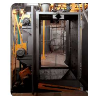
Blast Chamber Manganese Lining
